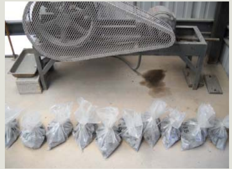
Sample Preparation Facility
