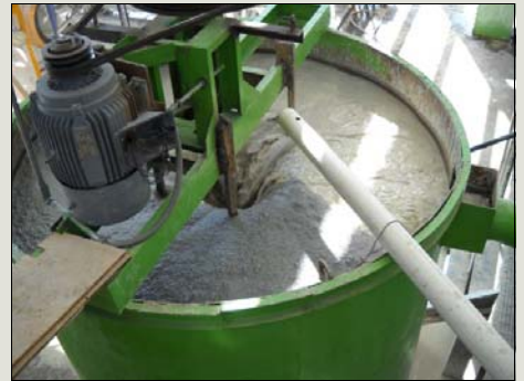
Flotation Conditioning Tanks
